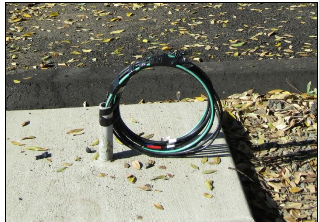
Figure 5 - Electrical Wiring for EV Charging Station at CIW
