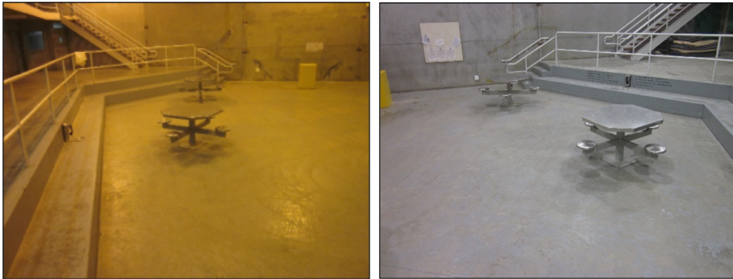
Figure 13 - High Pressure Sodium Fixtures vs. Energy Efficient LED Fixtures Before and After
