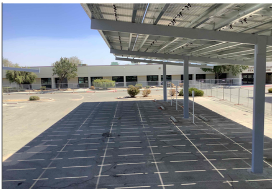
Figure 1 - Solar Canopy Installation at PVSP
