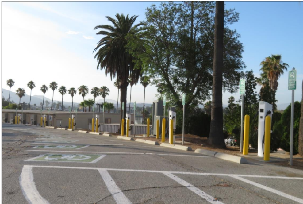
Figure 8 - Fleet Electric Vehicle Charging Stations - CRC
