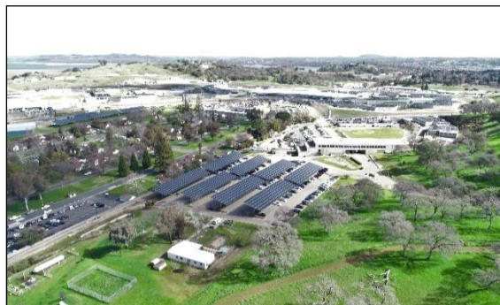
Figure 18- Solar Arrays - SAC
