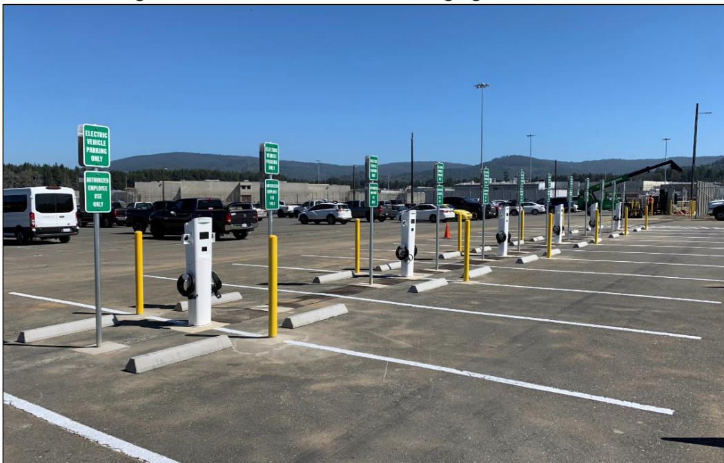
Figure 7 - Fleet Electric Vehicle Charging Stations - PBSP
