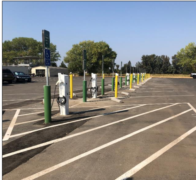
Figure 10 - Workplace Electric Vehicle Charging - CTC
